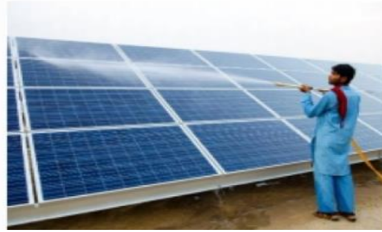
Figure 2: Water cleaning of PV panels (Bagnold 2012)
